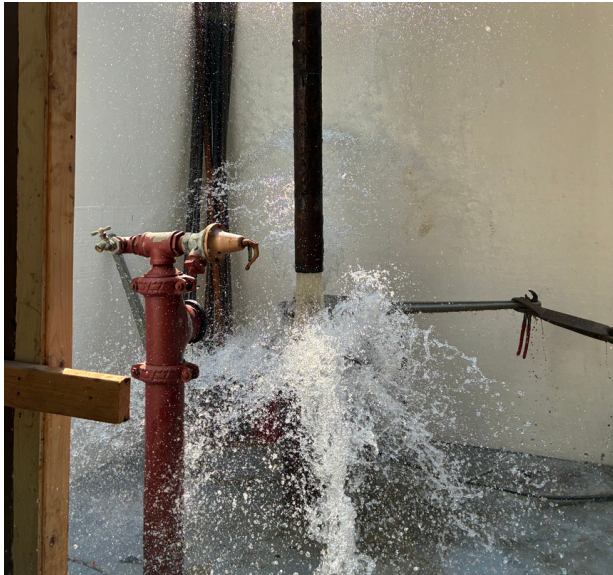
Water draining from pipe.
